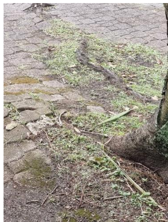
Footpaths damaged or displaced by the roots of large trees.
