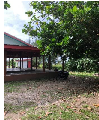
Figure 16: Overgrowth of trees is a hazard waiting to happen, in this case over the Are
