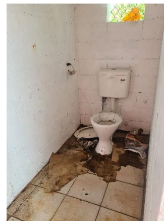
Public toilet next to the Catholic Cemetery in need of an upgrade.
