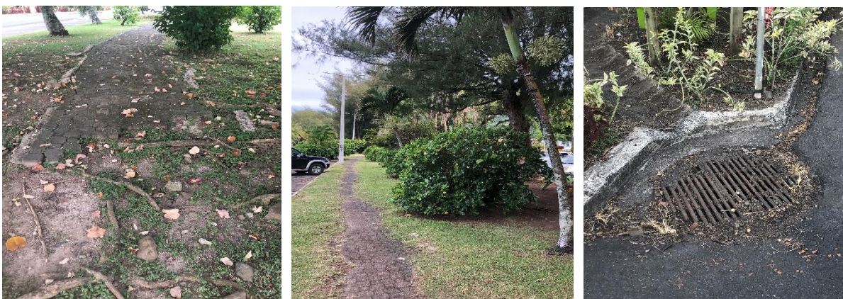
Figure 9: Some of the landscape characters identified; L-R. Damaged foot path by roots, footpath requiring maintenance and drainage systems around gardens.
